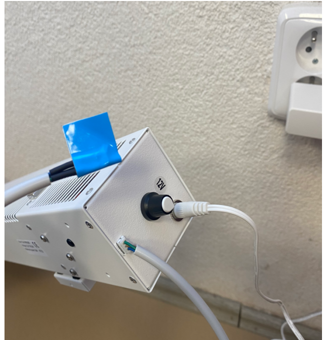
Pic.2 Temperature sensor connection
